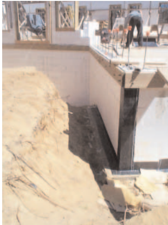
Figure 2. Twelve-inch-wide membrane strips reinforce vulnerable corner transitions and ensure a good bond over the cant strip.
