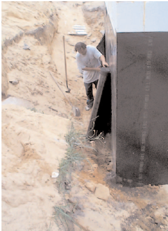
Figure 6. To direct ground water to the perimeter drain and protect the membrane from impact during backfill, fabric-filtered drainage mat is applied over the membrane.
