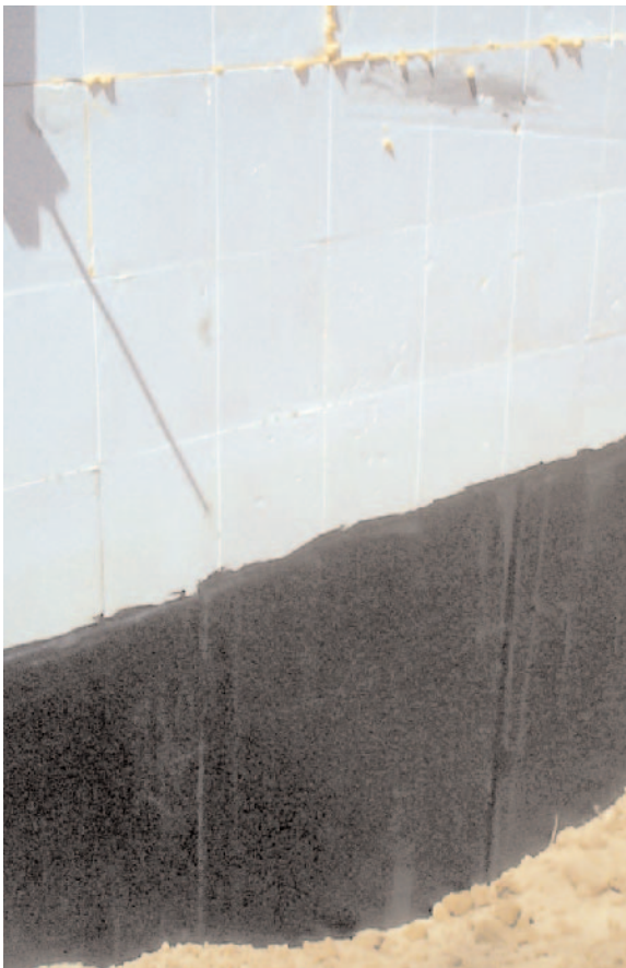
Figure 4. Membrane overlaps are pressure-bonded using a hand roller, then treated from bottom to top with proprietary sealant. Horizontal membrane terminations are caulked with mastic to complete the barrier system.
