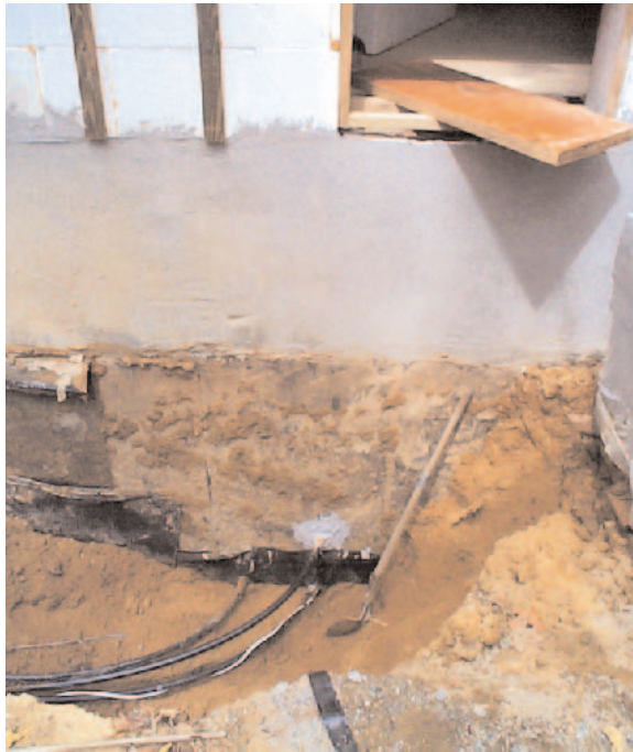
Figure 5. Water lines, drilled through the wall at a later date, are sealed with two-component urethane adhesive sealant, which cures to form a tough, elastic plug.
